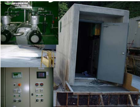
Vacuum station entry, with vacuum pumps underground
