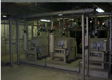
Inside of Vacuum- Station
