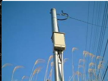
Relay unit on the pole
